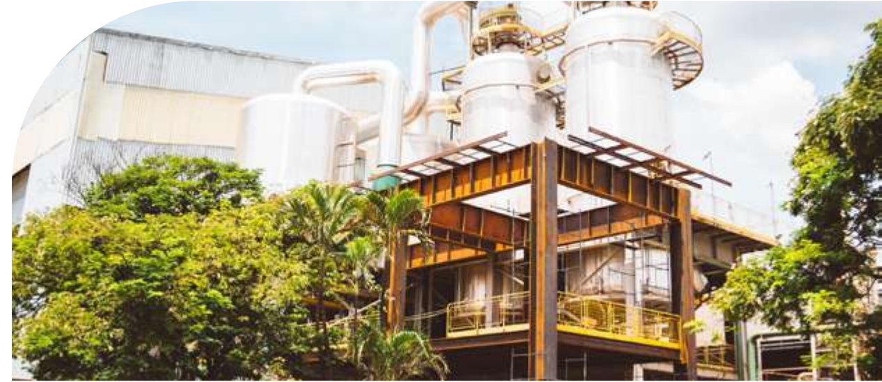
Vacuum pan and pre-evaporators, and, at the front, structure for new evaporators and vacuum pans for the 24/25 crop (Sugar Plant)
